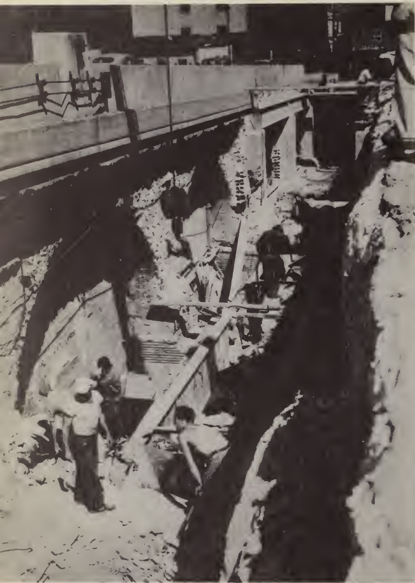
Arches of the old subway cut on the Manhattan side were removed preparatory to replacement with stronger arches to support traffic.
